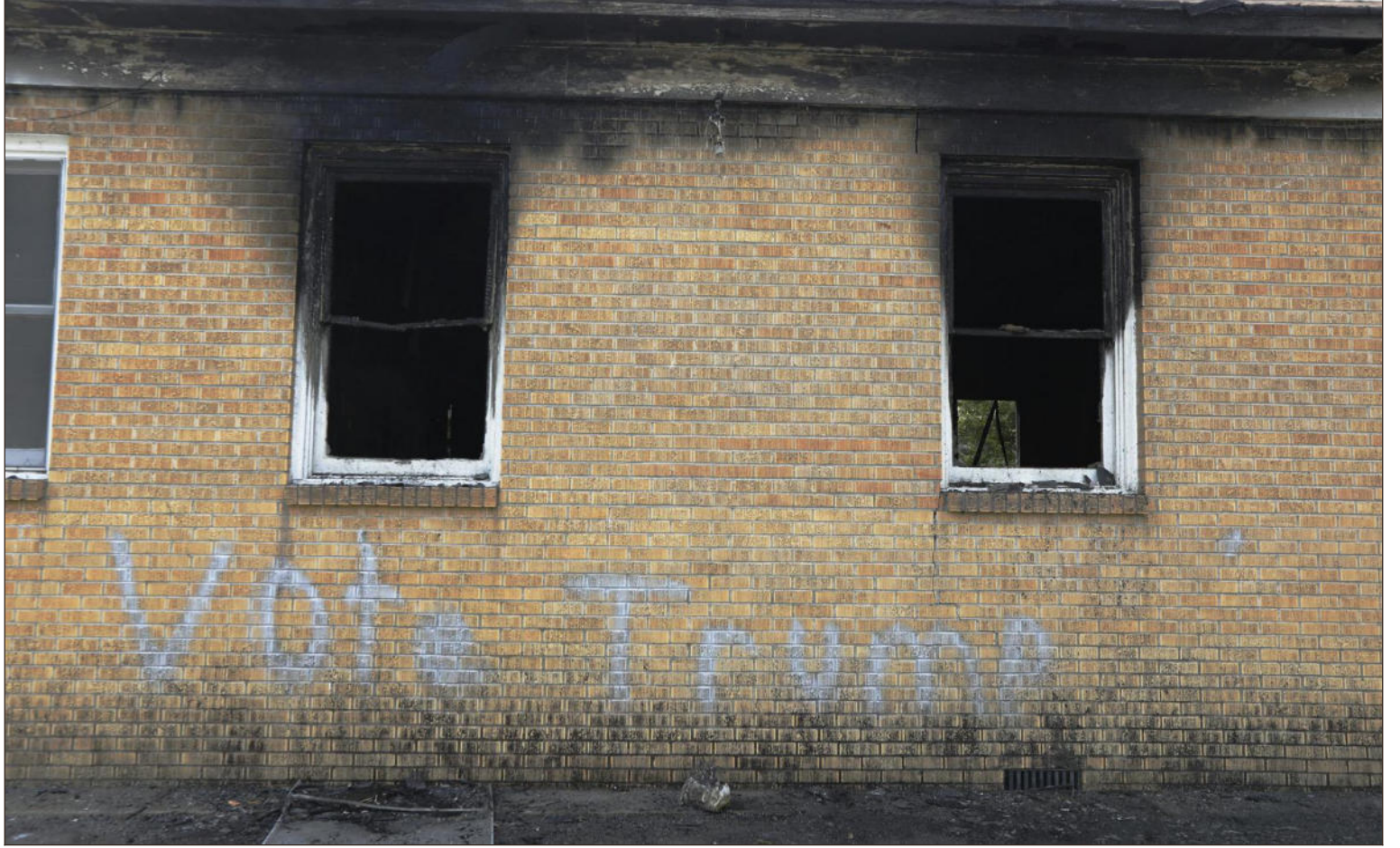
"Vote Trump" is spray painted on the side of the fire-damaged Hopewell M.B. Baptist Church in Greenville, Miss., in November 2016. But authorities discovered that it was done by one of the church's black parishioners, over a dispute within the congregation.
